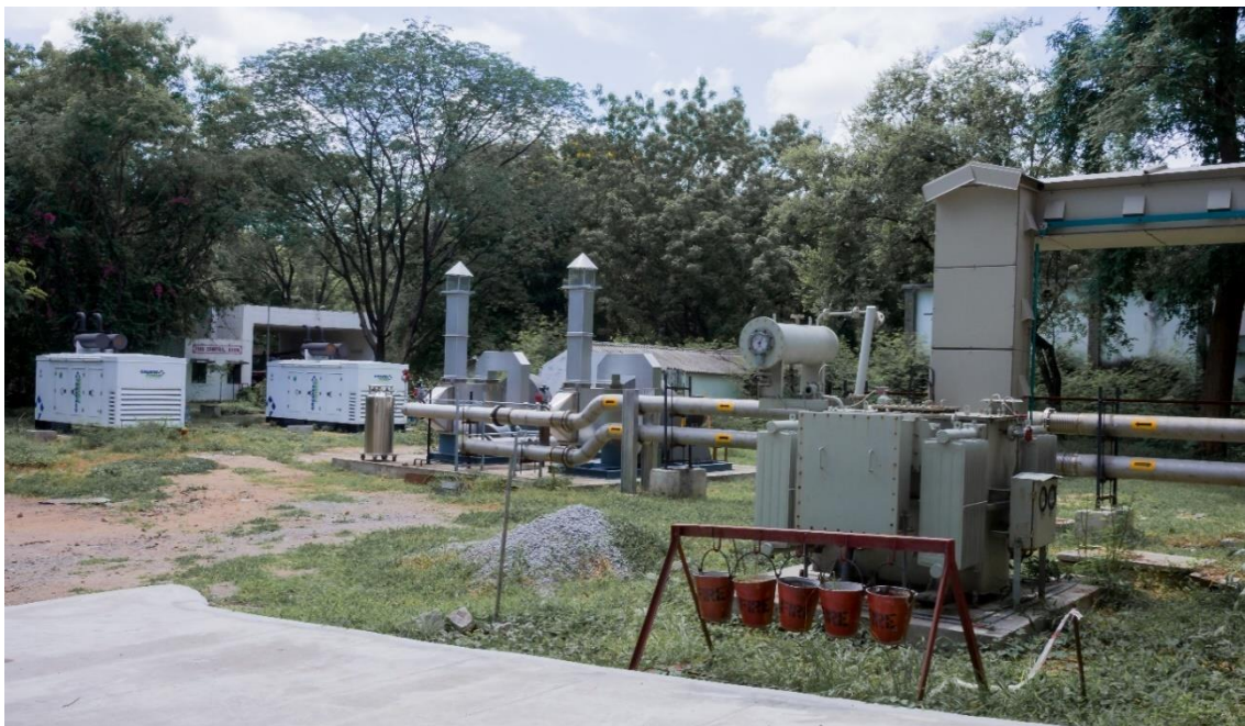
Fig. 4: DG Sets, Nitrogen Blowers and Transformer for Rotor Test Rig
