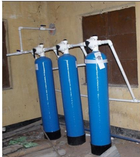
Treatment unit within a room in the school
