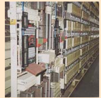
Automatic Telephone Exchange
