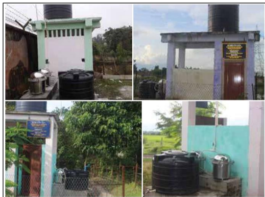
Water Filtration Units Installed at SC/ST villages, Imphal, Manipur
