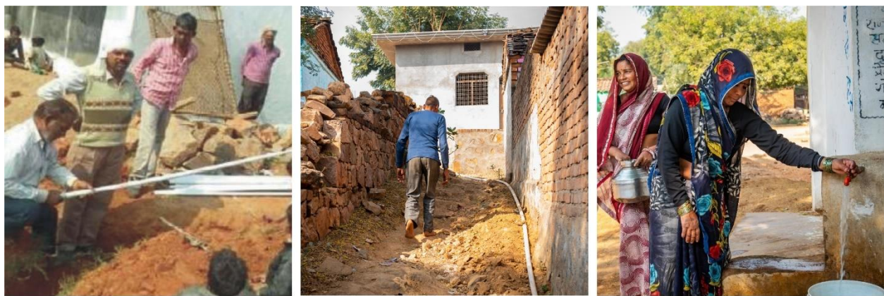
Community engagement in installing solar powered pumps and laying down pipelines to supply water up to community water stand posts, ensuring clean water for all.
