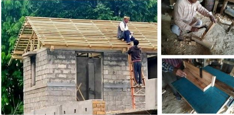
Shri Satya Singh Panwar's unit – timber shingles and truss roofing services at Kamad, Uttarkashi
