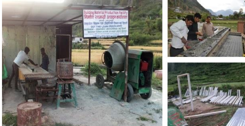
Shri Santosh Semwal's unit - concrete based pre-fabricated building elements unit at Matli, Uttarkashi
