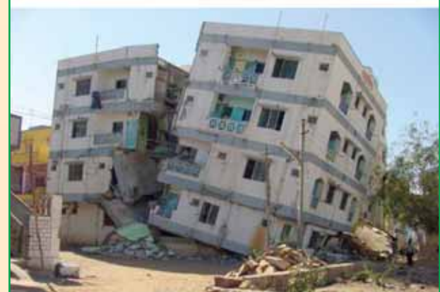
(b) Collapse of reinforced concrete columns (and building) during 2001 Bhuj (India) earthquake
