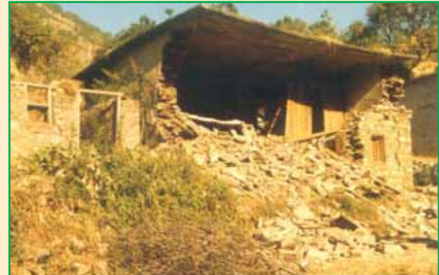
(a) Partial collapse of stone masonry walls during 1991 Uttarkashi (India) earthquake
